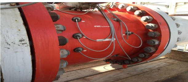
Figure 2: Photo of the pipe under study with the ultrasonic devices
